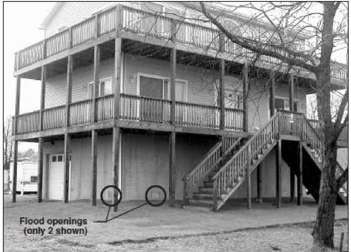
Figure 3. Full-height solid perimeter walls surrounding garage and storage area (only two openings visible)
